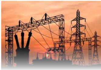
Power System Studies
