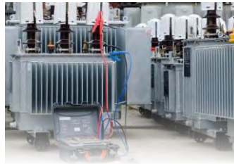
Electrical Network Health Analysis
